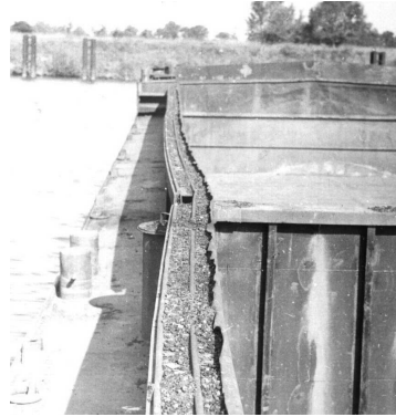
Fig. 10. Example of macro notch of deck transom of river barge BP-500
